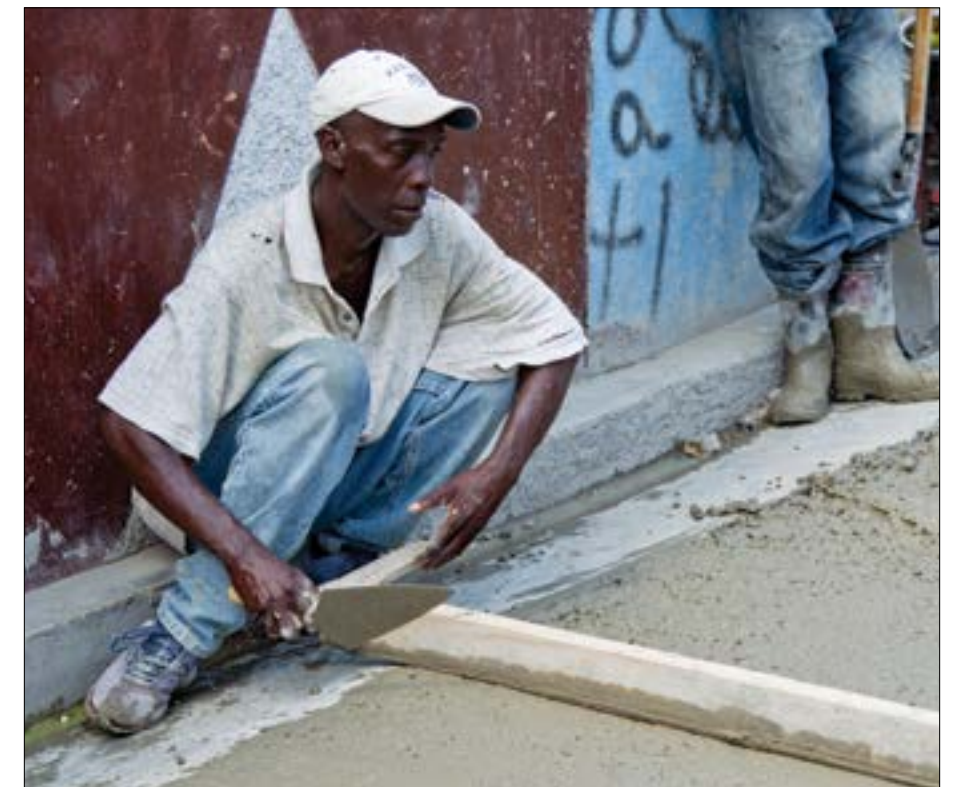
A labourer in Haiti works on a UN sponsored development project. In 2011-12, CIGI's Global Development Program focused on identifying innovations that support sustainable development and facilitate a shift to a more equitable delivery of global public goods.
